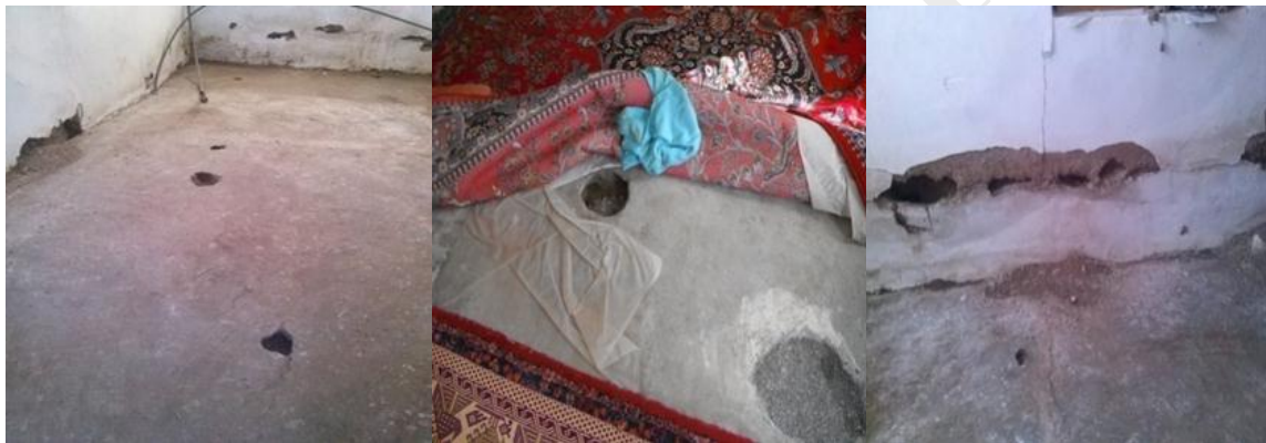
Fig. 2. Effects of rodent infestation to houses in Najaf Abad village; ruined floor of residential houses
